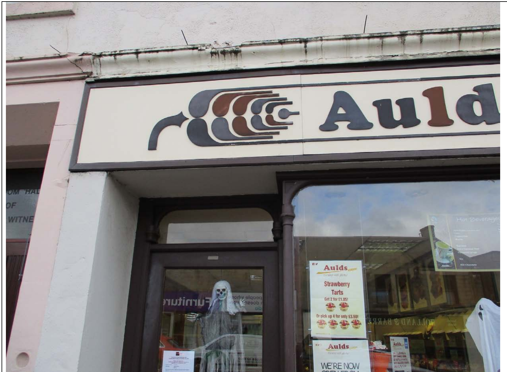
Photo 9 – Fascia board ( taken 12/10/2017)
