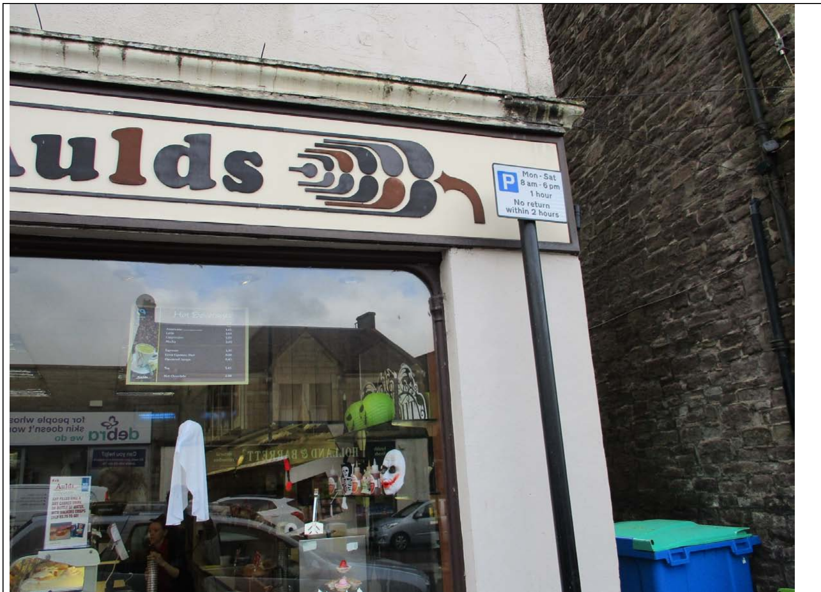
Photo 10 - Fascia board ( taken 12/10/2017)
