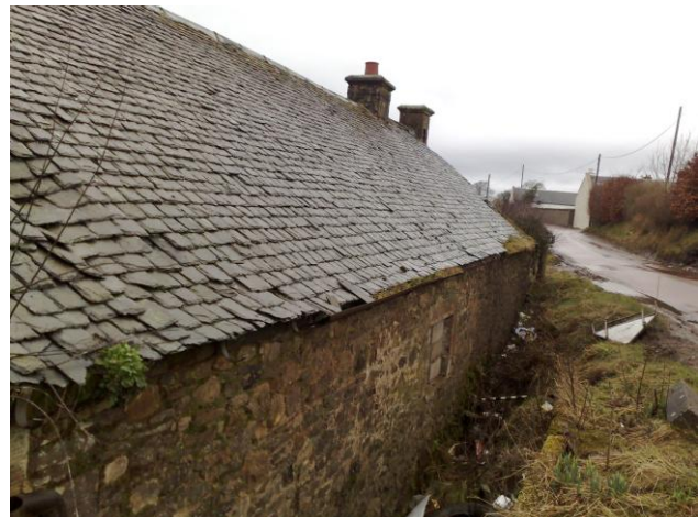
Bankfoot 2007 - Clearly derelict at the time of visit.
