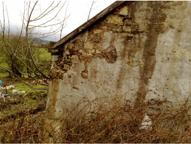
Bank foot 2007 - tree growing out of the wall of the house.
